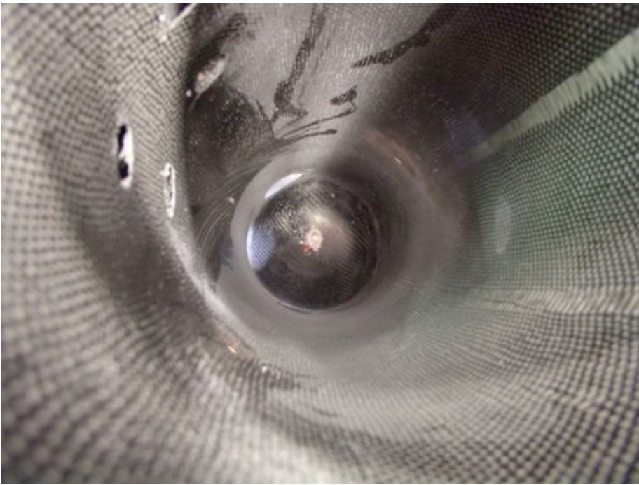
Picture 5: The hole is made (internal view) Make sure to clean the container.
